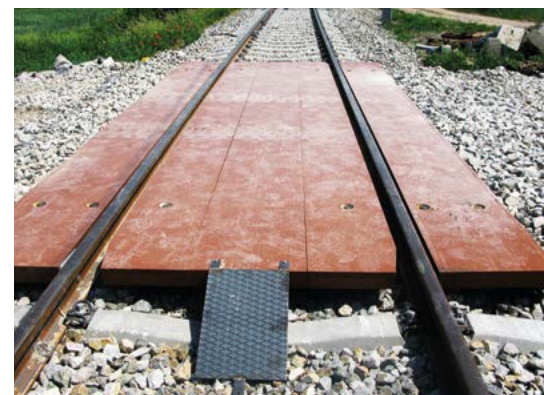
Fig. 4: ÖBB, Protectors in the mountains, synthetic wood level crossings
