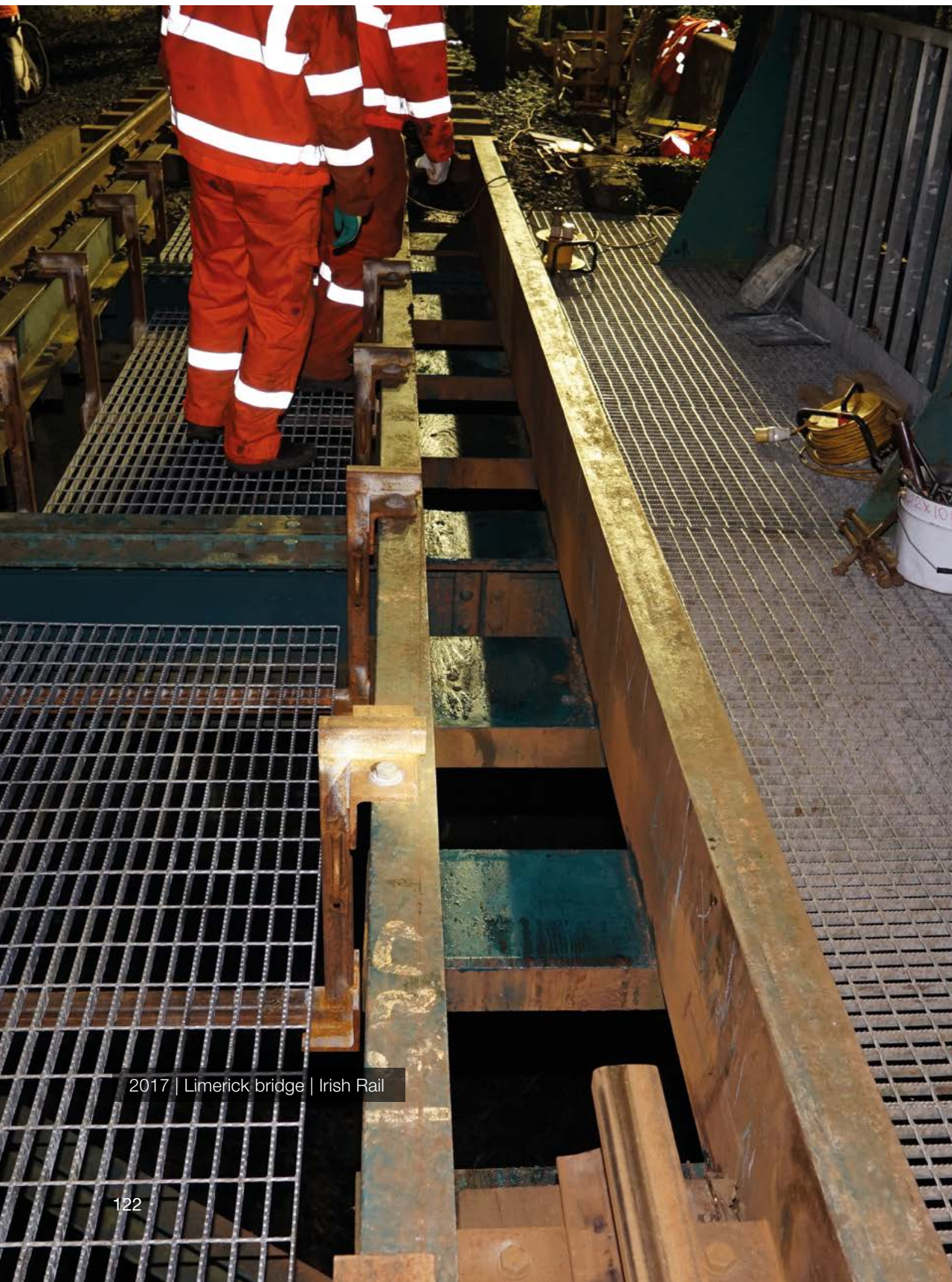
At Ube Bridge in Limerick, FFU Longitudinal Bulks are running under the rail and resting on cross steel bridge girders.
